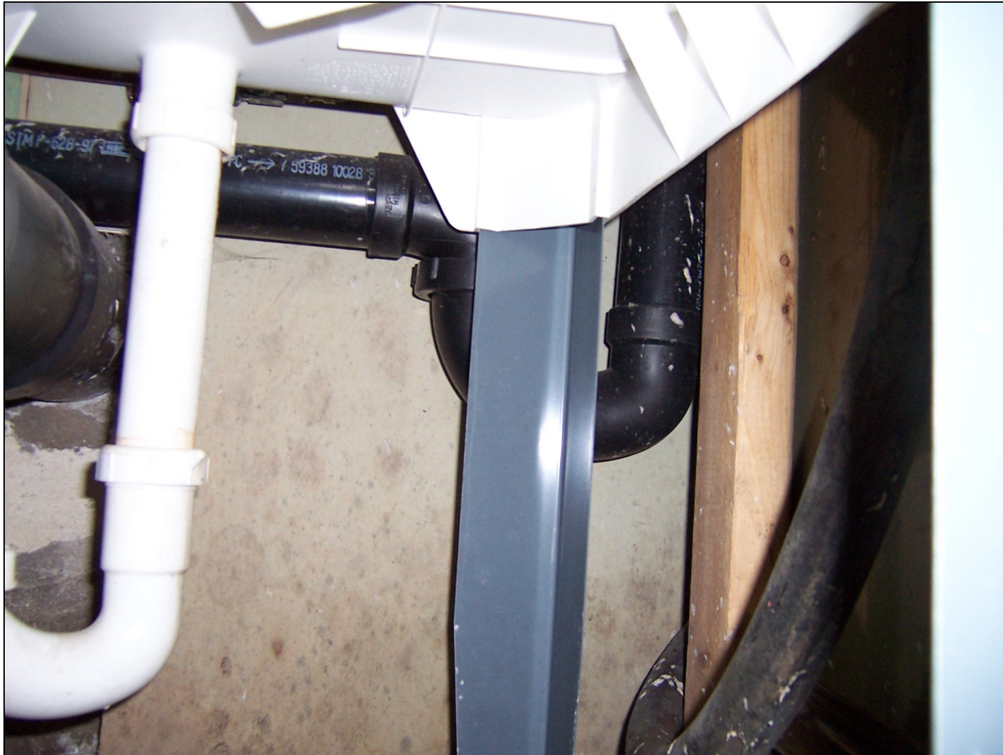
Figure 12: Washer drain not vented
