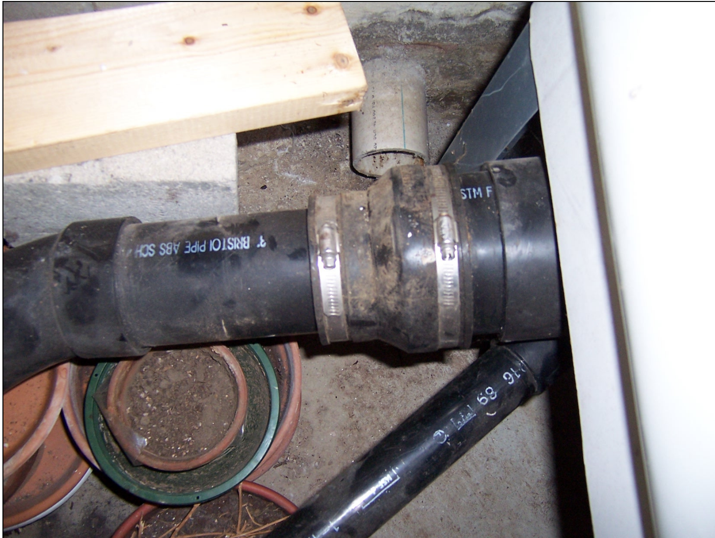
Figure 4: 4 inch to 3 inch reducer in drain line
