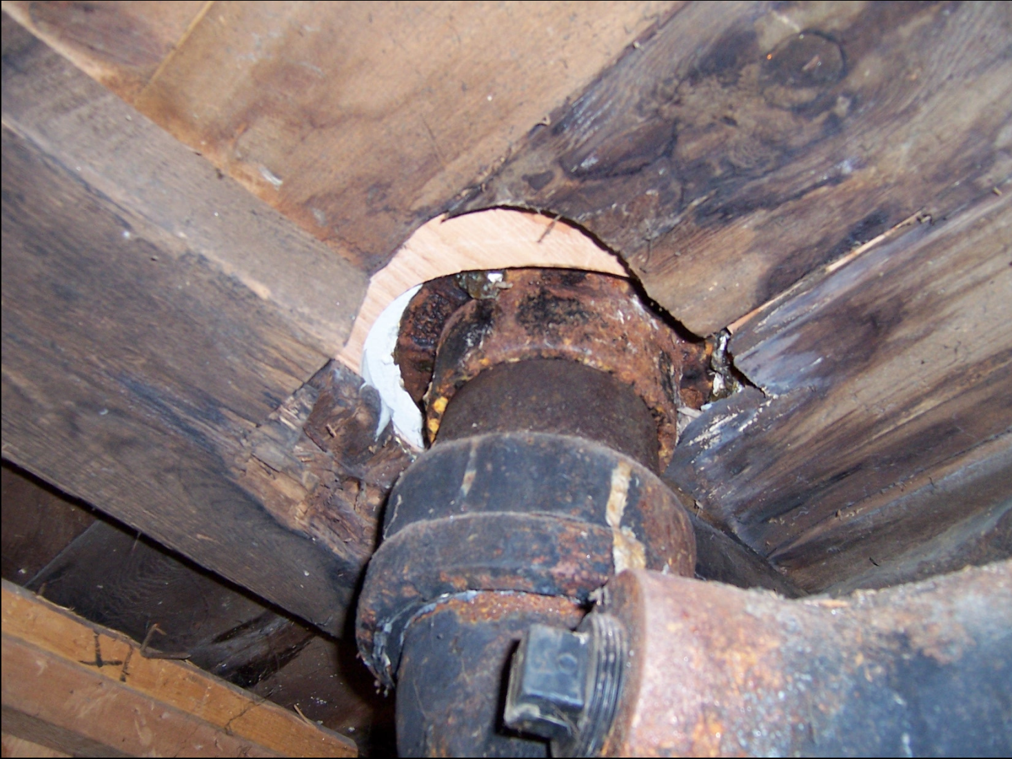
Figure 8: Floor cut away under toilet allows toilet to shift
