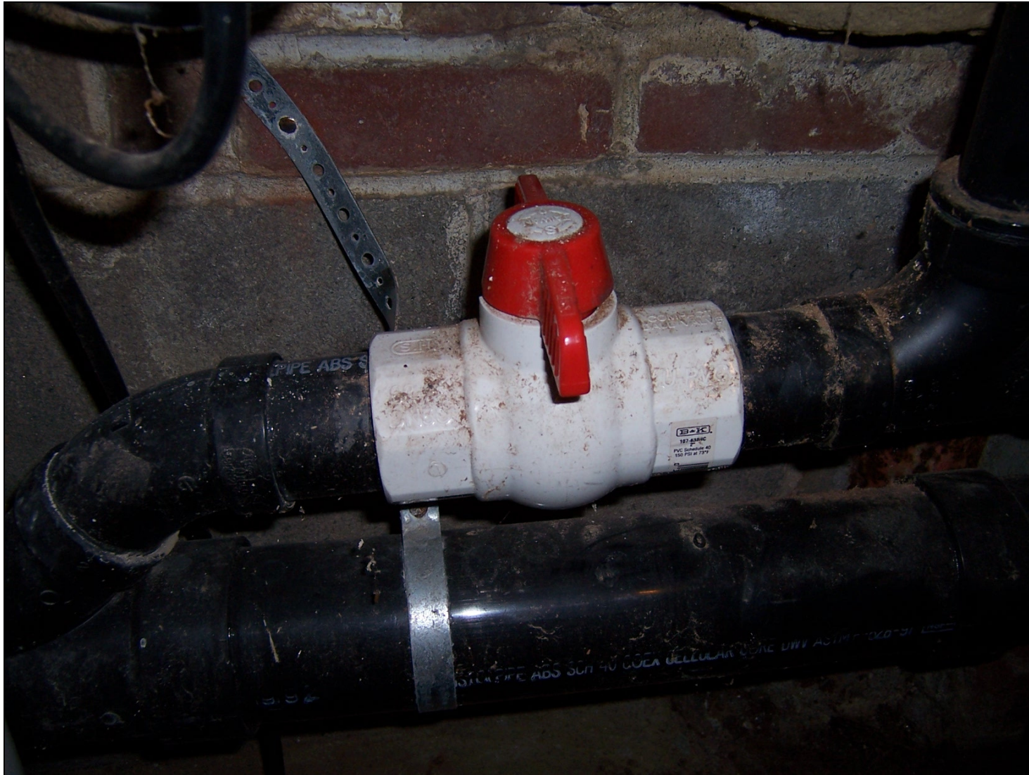
Figure 3: 2nd ABS drain valve needs to be removed or replaced with PVC
