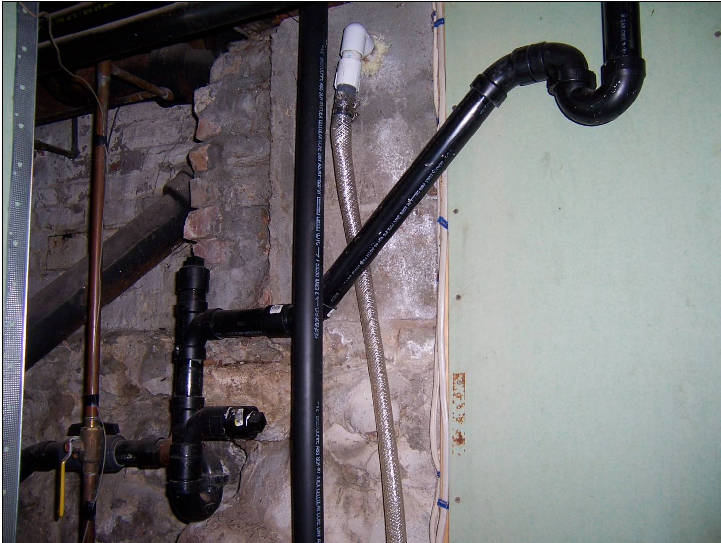
Figure 11: Sink drain below floor and double trapped
