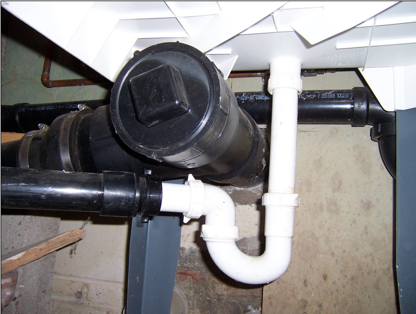
Figure 5: ABS mixed with PVC, no Vent and illegal pressure fitting, also pictured is the misplaced cleanout in drain line
