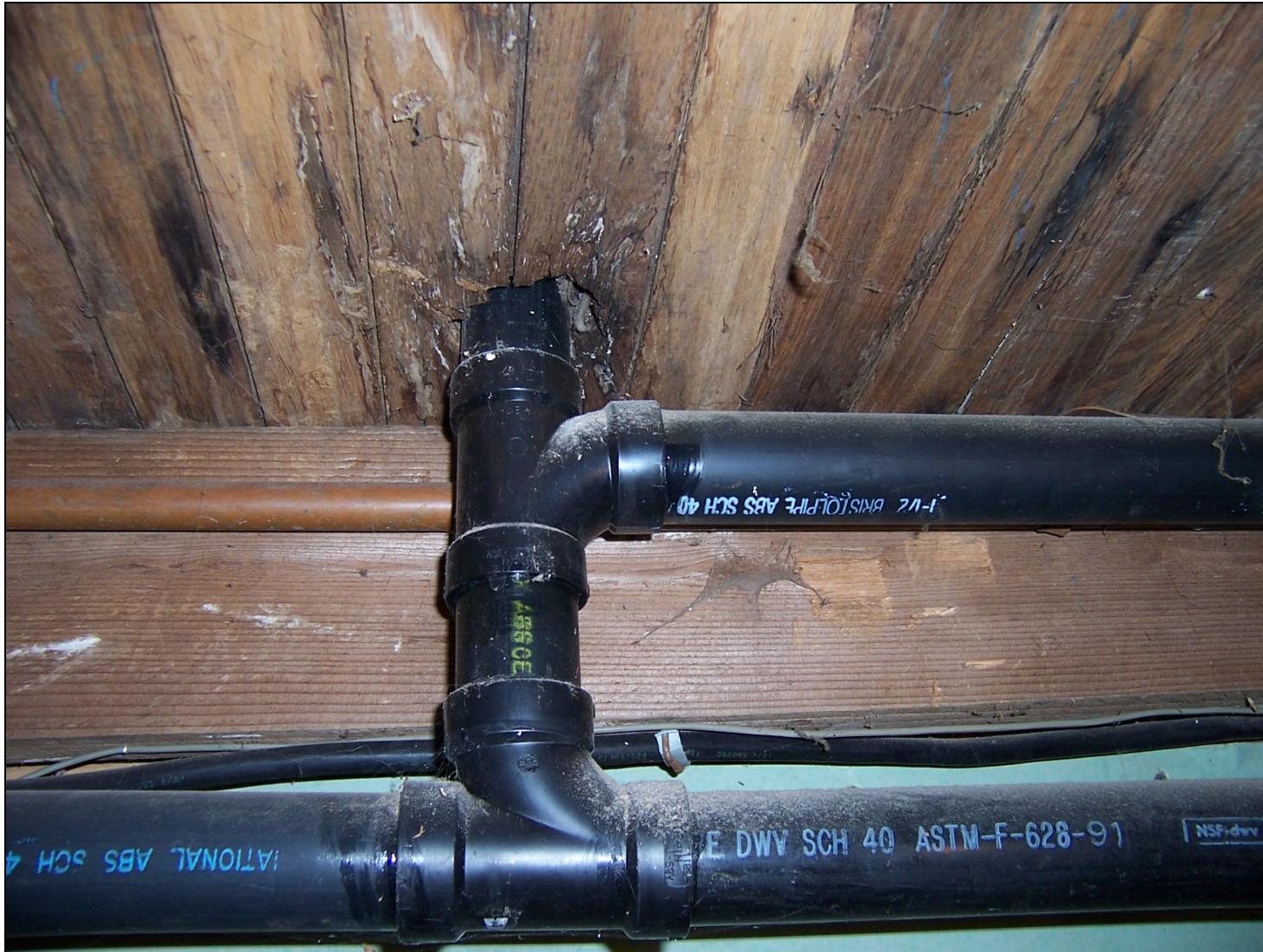
Figure 1: Fitting installed upside down
